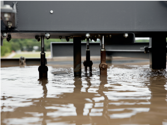
06/ FULL-LENGTH VALVE BRIDGE
